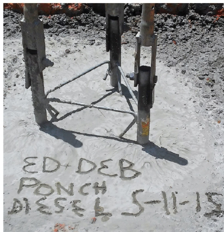
Eddie and Deb celebrated the completion of the tower's base by marking their names in the still-wet cement — Eddie's dogs Ponch and Diesel got special billing as well.
